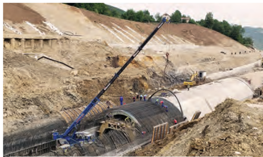
Koridor Vc, dionica Klopče-Donja Gračanica, obilaznica oko Zenice, cut and cover tunnel
